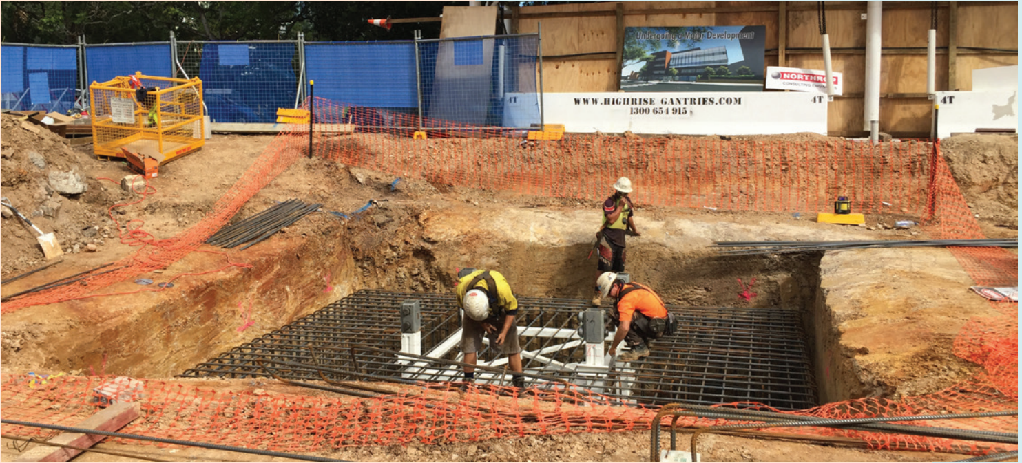
TOP TO BOTTOM: GLOBAL BUILDING COMPANY COCKRAM BEGINS CONSTRUCTION ON STAGE ONE OF THE HOSPITAL EXPANSION
